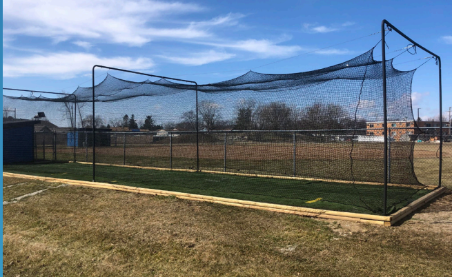
New softball batting cages constructed by the XCS Facilities Department at Xenia High School. (February 2021)
